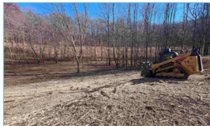
Contractor Josh Delozier with Grounded Land Solutions operating a gyrotrac in the Hall Farm prepping a native grasslands initiative 15 seed mix. Photo by Steve Ward
