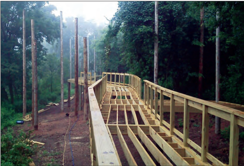
A boardwalk is under construction from the education center on Hall Rd. to the aviary.
