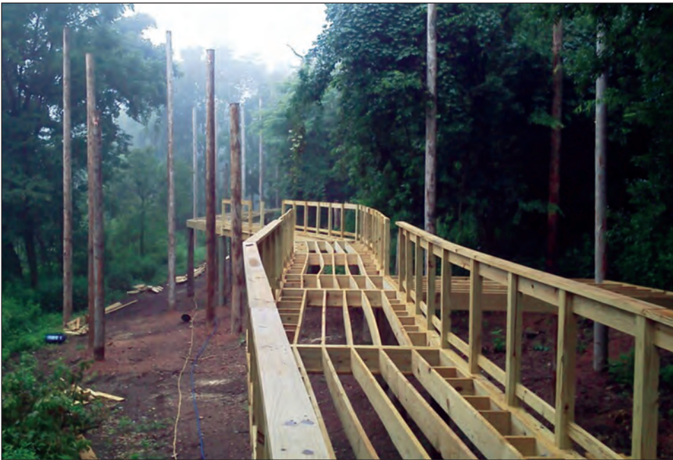
A boardwalk is under construction from the education center on Hall Rd. to the aviary.
